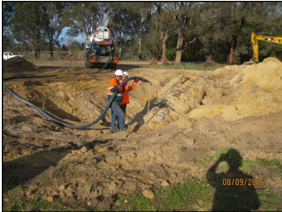
Photo 5: Photograph of the removal of liquid sludge from the UST, facing south.
