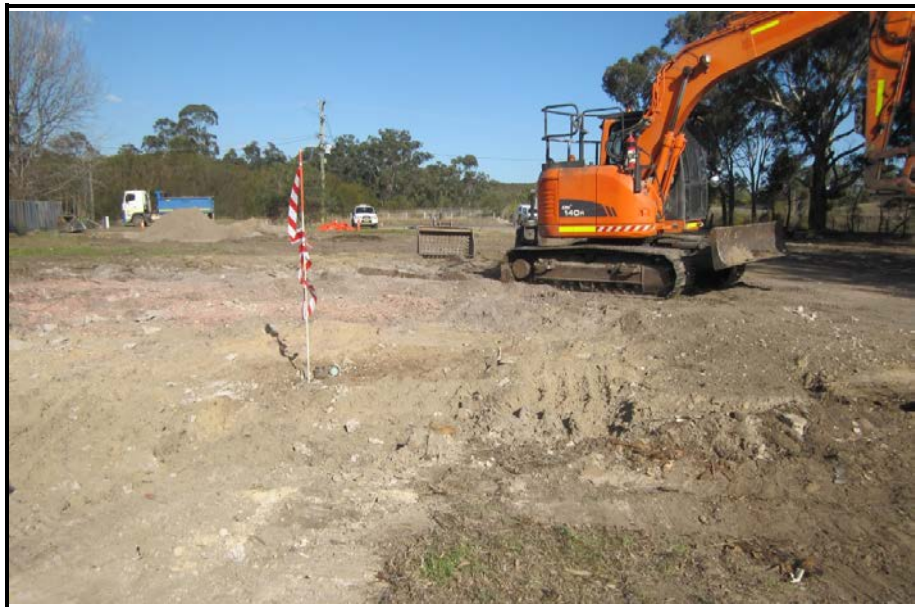
Photo 2: Flag showing location of the UST following demolition of the shed, facing east.
