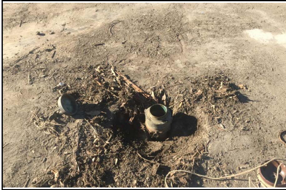
Photo 3: Photograph of the dip pipe, indicating the presence of the UST.
