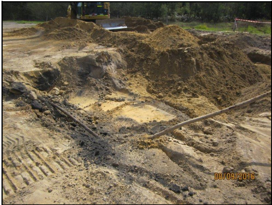
Photo 10: Photograph of pipework to chase out and black coal washery reject subbase.
