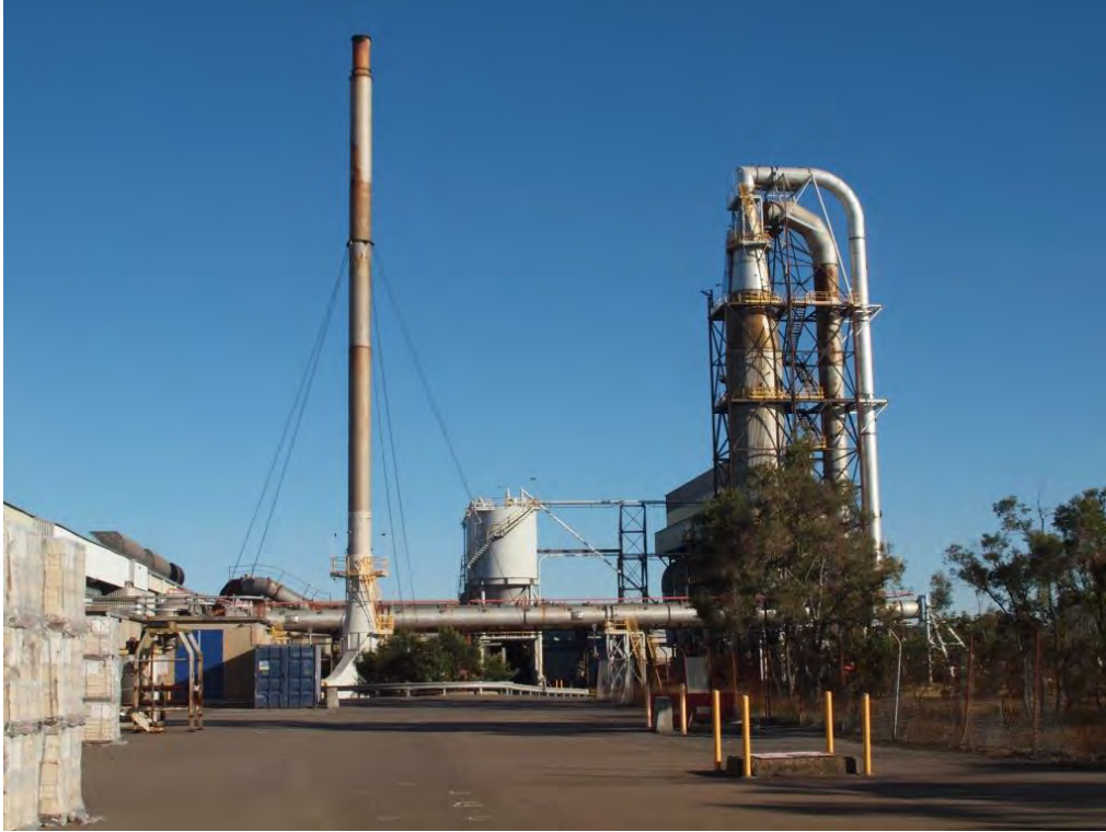
Plate 7 Looking west to Scrubbing Plant
