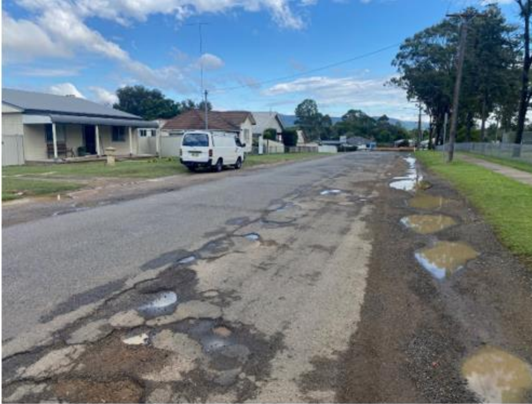
Figure 3 – Anderson Avenue Paxton – Pre-works Photograph
