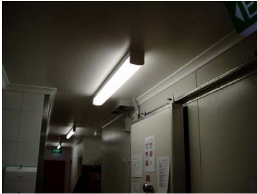
Picture 3: Light fitting with diffuser cover
